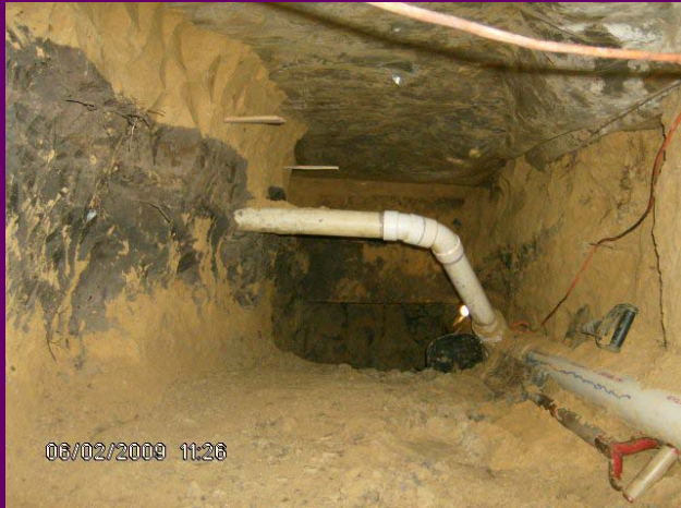
Tunneling work being done at Port Neches Elementary for new plumbing lines
