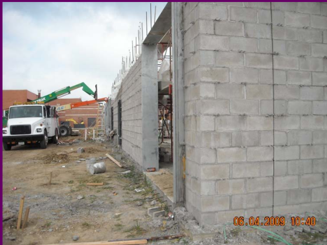
Block walls are being installed at the CATE area of New Building
