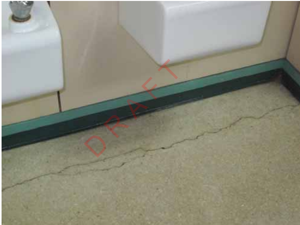
PHOTO VBES2 - FLOOR CRACKS
